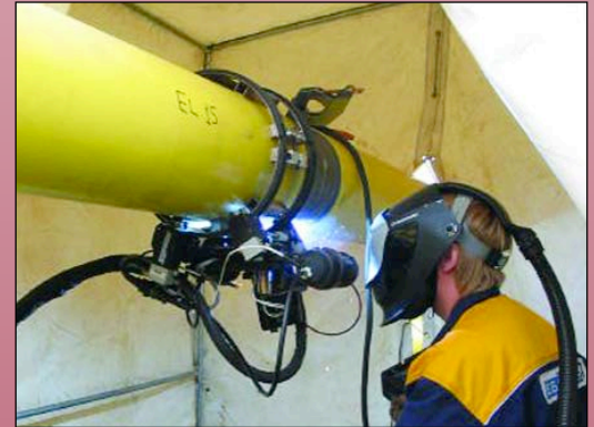
27cm (10") Gas Pipeline – Estonia
